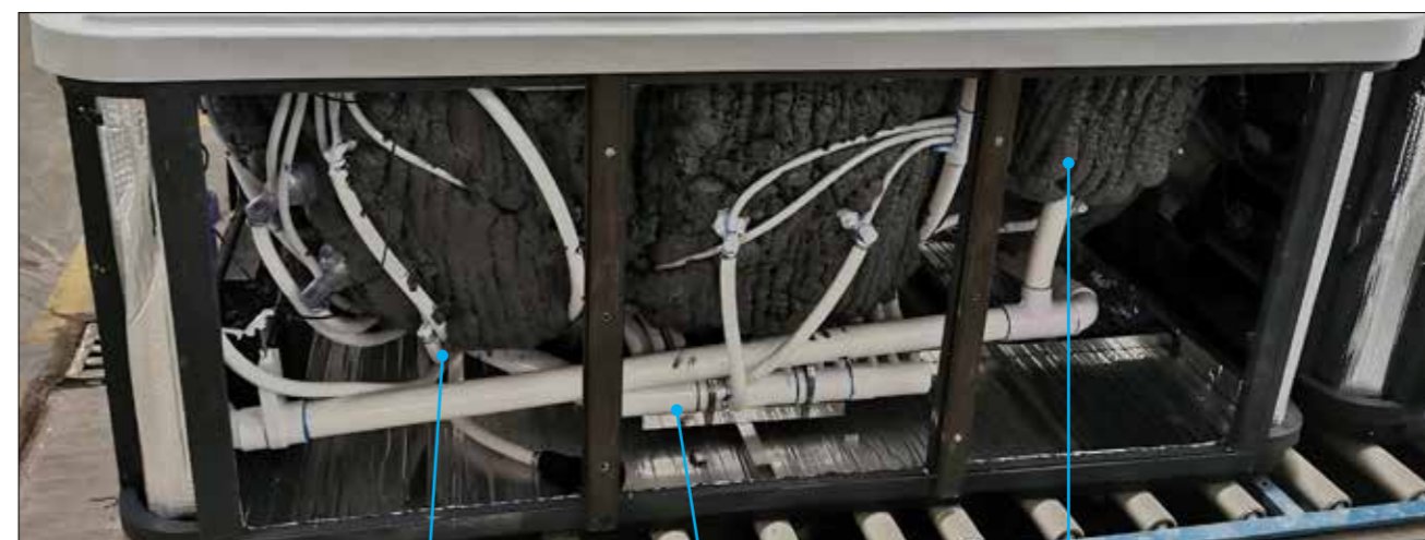
Slice Valve Manifold Black out insulation
